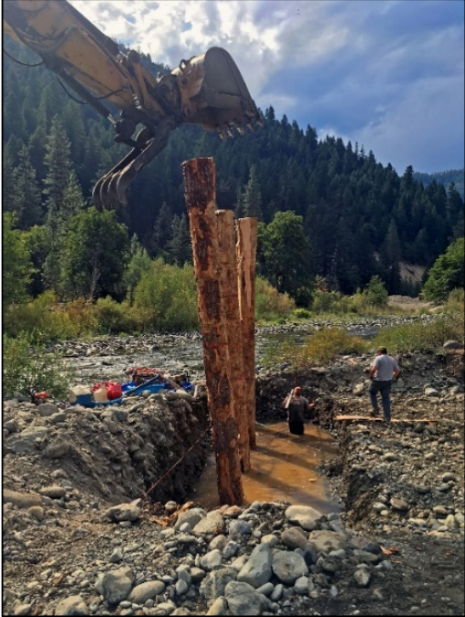
Image 4: Mid-Bar Channel engineered log jam structural uprights (i.e., piles) being installed. Summer 2019.
